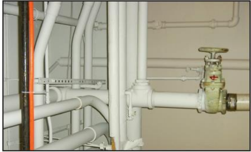
Piping and plumbing systems
