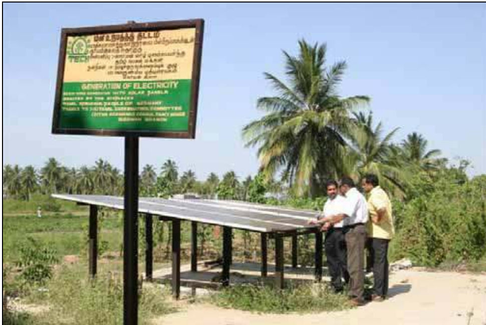
Fig. 2. Solar panel installed in NE-SL
