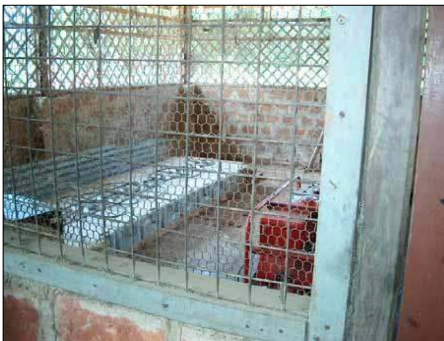
Fig. 4. Battery Storage System
